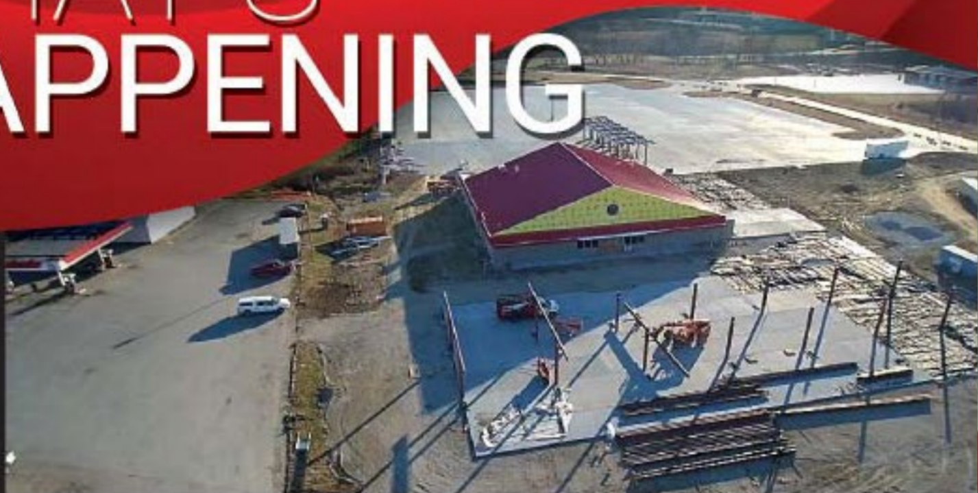
Aerial view of the construction process of the new Sapp Bros. Travel Center in Harrisonville, MO
